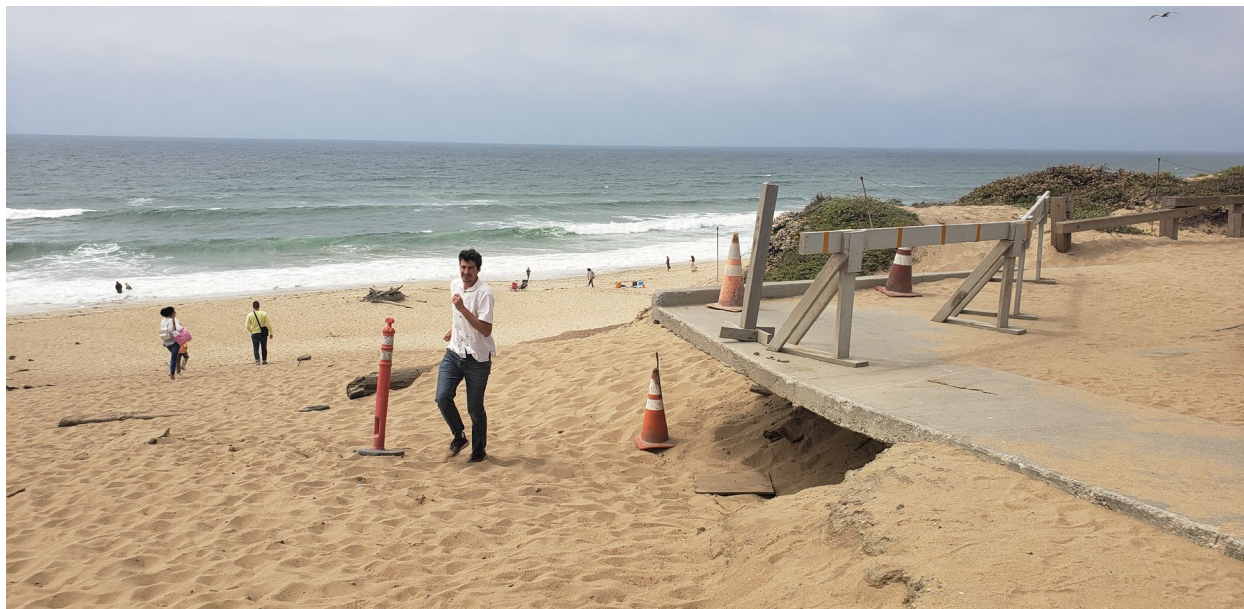
Figure 6-4. Parking Lot Erosion at Marina State Beach (July 2019)
