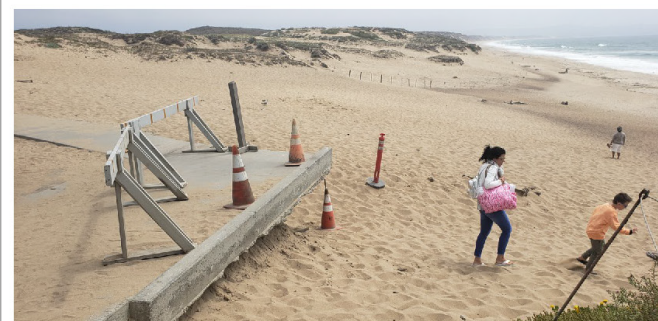
State Parks manages the Marina State Beach parking lot and coastal access amenities which is currently being undermined (photo left).
